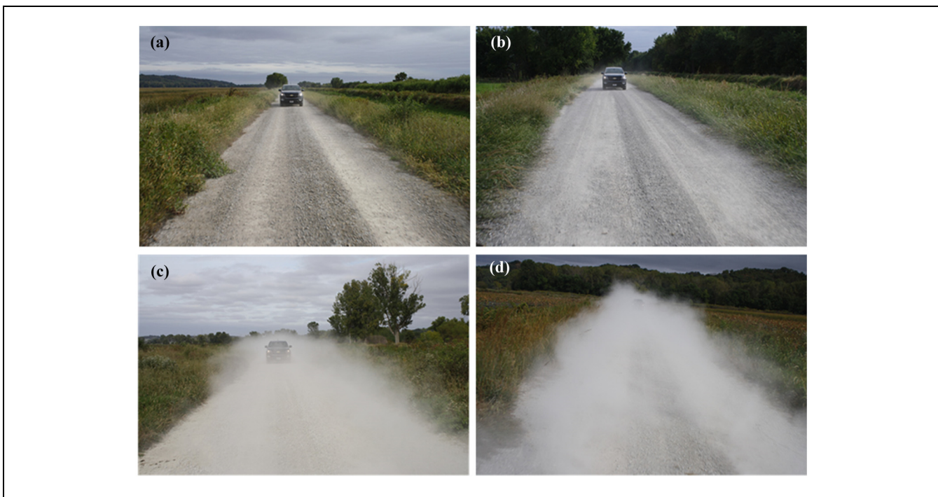
Figure 3. Representative dust levels 15 months after original product applications (5 months after maintenance application of EnviroKleen®): (a) durablend-C™-treated section; (b) EnviroKleen®-treated section; (c) untreated control section; (d) an adjacent road section on the auto tour loop that did not receive new surface aggregate or chemical treatment as part of the study, shown for reference. Photographs were taken from the back of a passenger truck traveling 40kph (25mph). Photo credit: B. Kunz, USGS.
